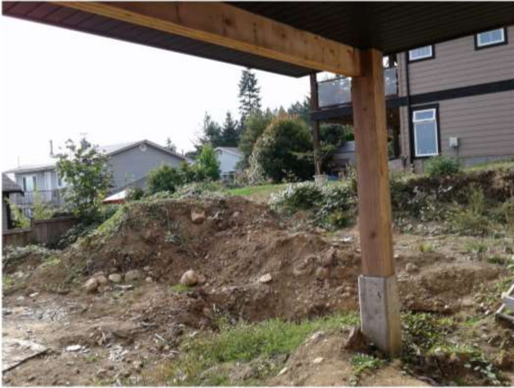
Figure 5: Southern Property Line Proposed to be reinforced with a Retaining Wall, Looking South from Under the First Floor Deck
